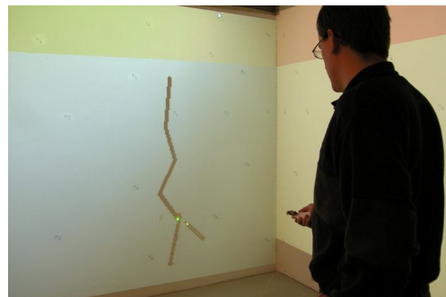
Figure 10 Tracing the line of a crack in the building fabric
